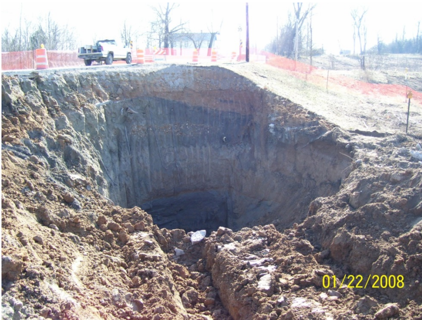
Huge Sink Holes
